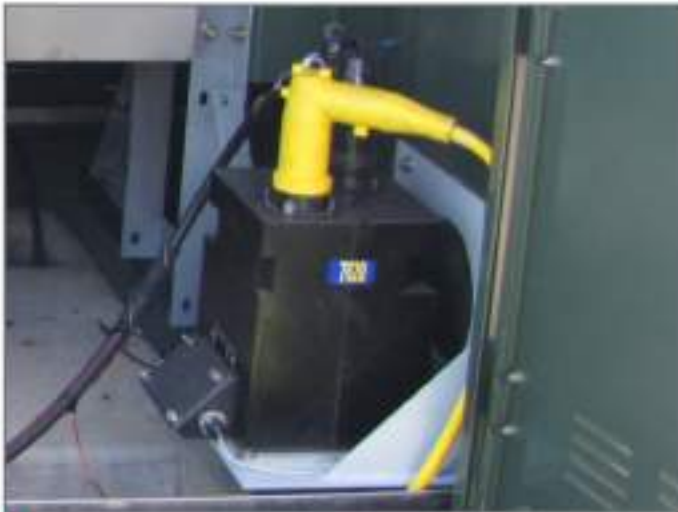
▲ Example of integrated external transformer
