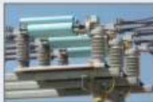
System Protection Equipment
