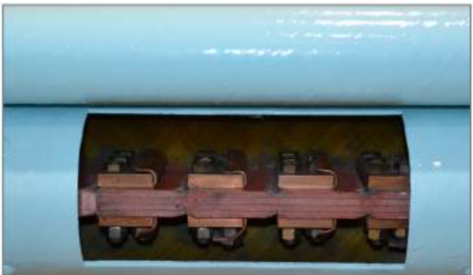
▲ Close up of the severed main conductor and melted current limiting element of a 3000A (double bus) CLIP after interruption.
