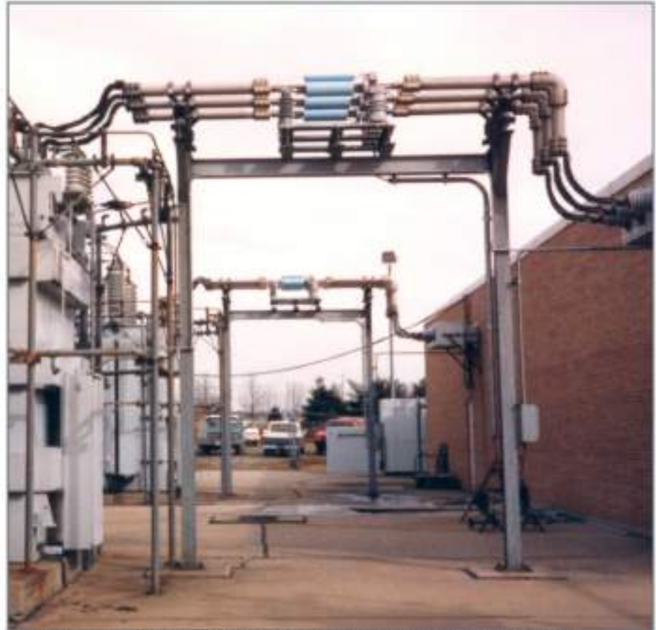
▲ 5.5kv, 3000A CLiPs protecting the utility from a small cogeneration plant.
