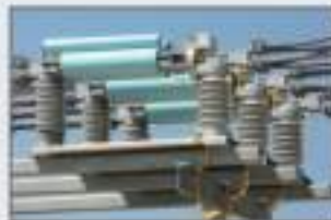
System Protection Equipment
