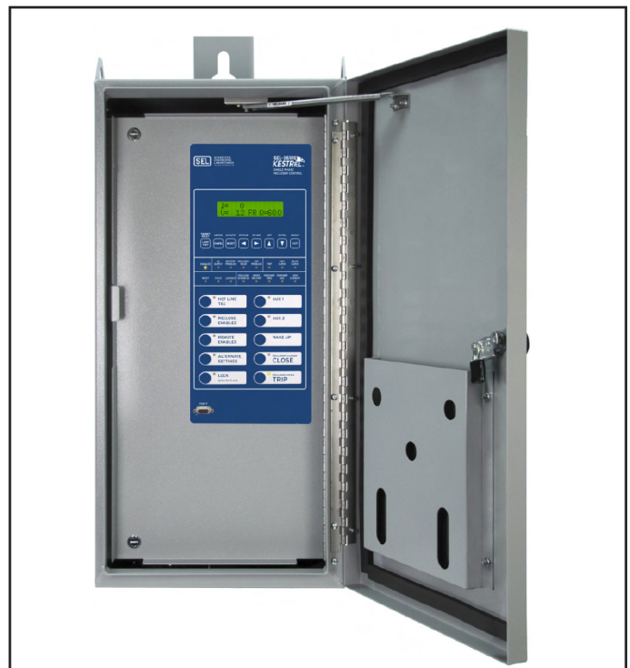
▲ Schweitzer's SEL-351RS Kestrel front access control with conventional swing panel enclosure. Swing-up style door also available.
