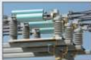
System Protection Equipment
