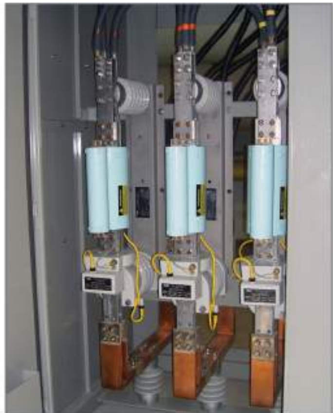
▲ CLiP protecting a methane fueled co-generators in a sewage treatment plant.
