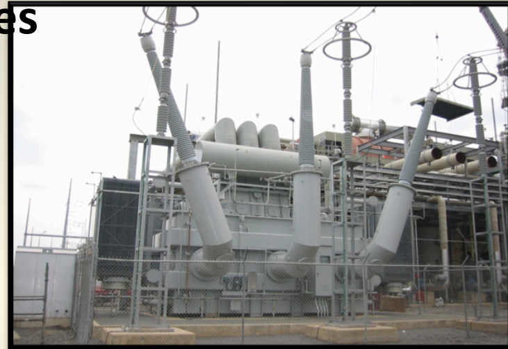
NEPCO El Dorado 18/525kV 315MVA GSU Year of 2001
